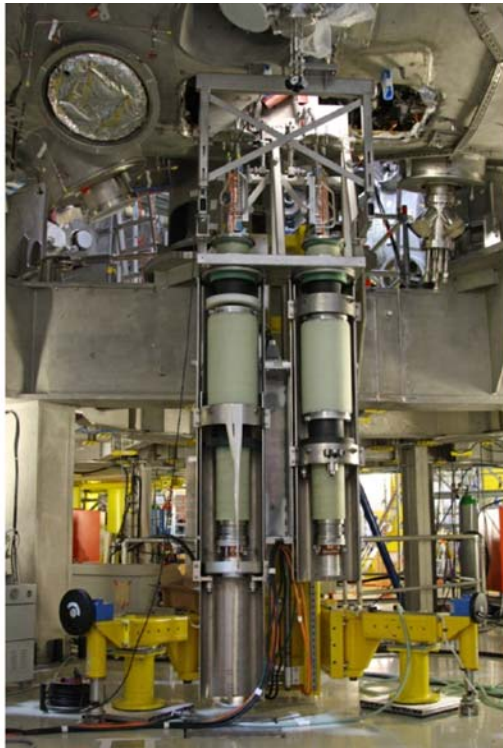
Fig. 4. Current leads for the superconducting coils. Photo: IPP, Beate Kemnitz
